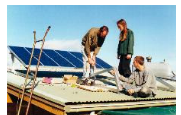
Helping Dad install the new solar panels. Thomas, now 17, monitors the system.
